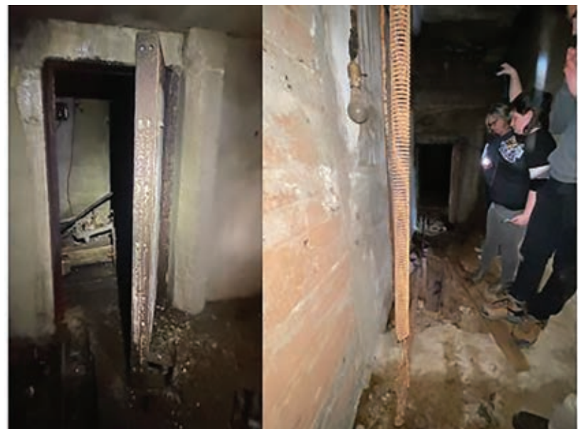
Basement steel and concrete door that leads to safe room tunnel No. 2-courtesy of Harbor Springs Museum
