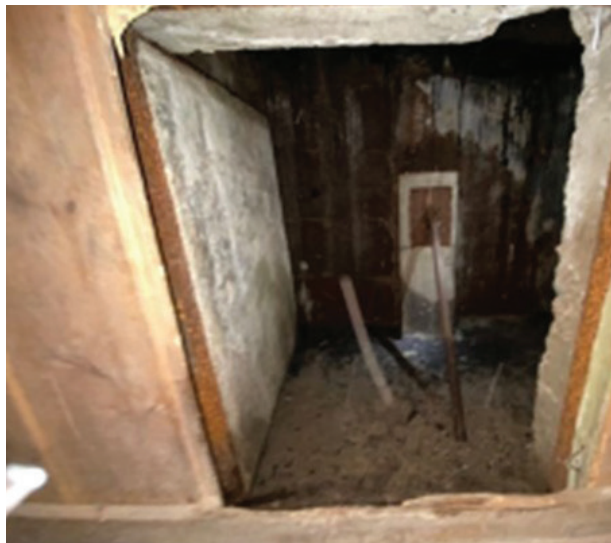
Opening in bathroom to the safe-room tunnel No. 3 and ventilation tunnel. (courtesy of Harbor Springs Museum)
